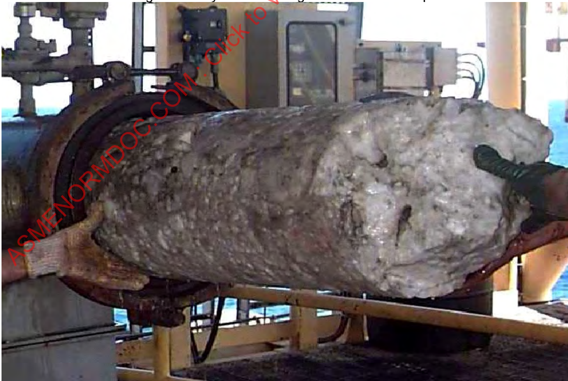
Fig. 9.1-1 Hydrate Blockage in a Section of Pipe
